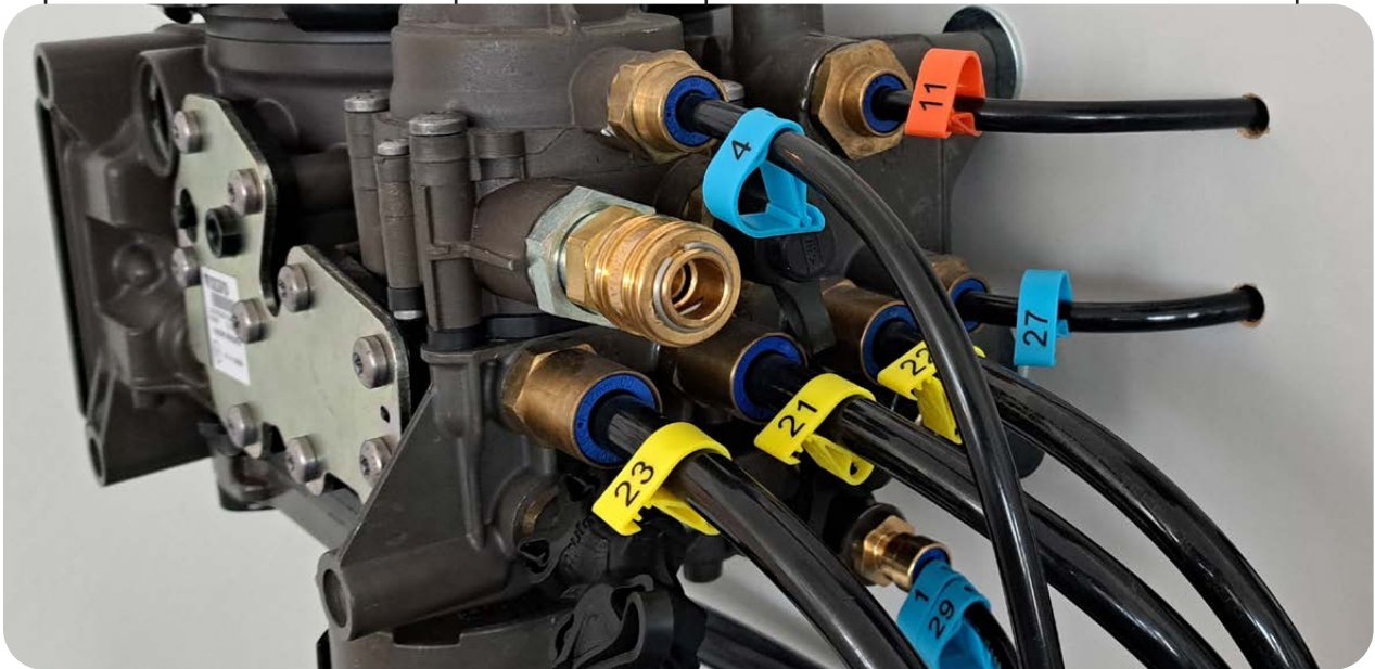
The pipe markers clearly identify each line.
